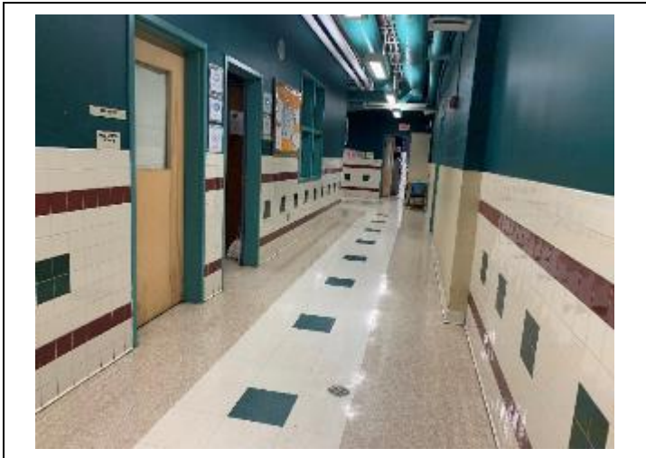
13. Hallway with wall tile adhesive and grout. No asbestos detected. ACMF flooring mastic below 12" Tile.
