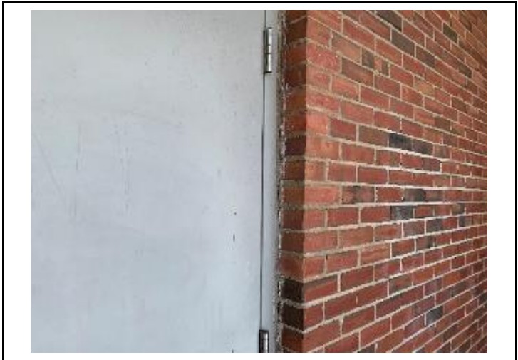
2. ACBM remnant door caulk. Assumed to be around all doors on original brick structure.
