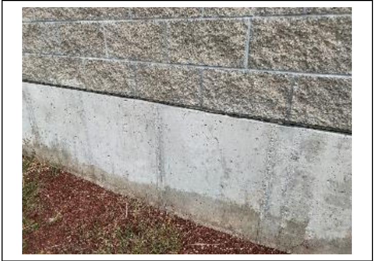
4. Black sealant on addition flashing on the base of the exterior wall. No asbestos detected.
